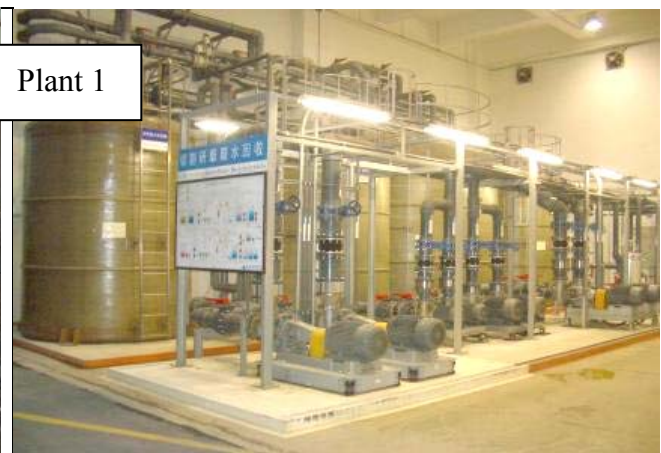
Cutting and grinding waste water classification and tubing for collection and recycling
