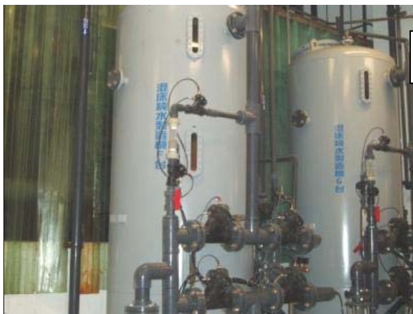
Pure water system in mixed bed recycling to supply RO water from soft water area
