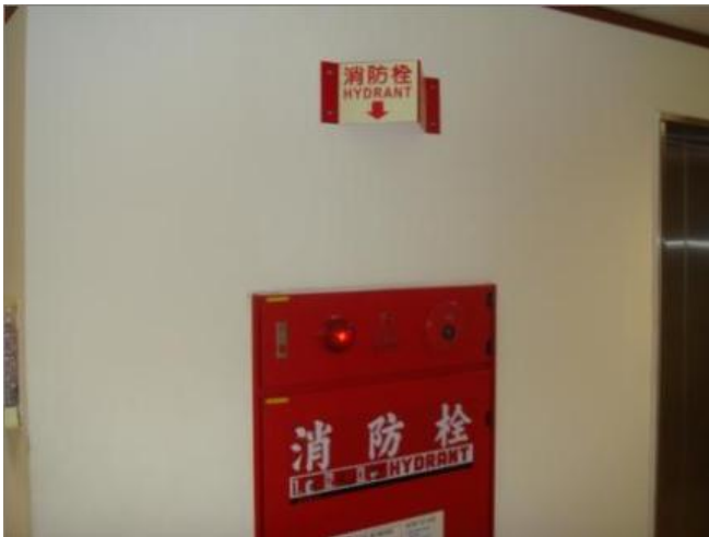
Fire hydrant with protruding signs for reminder.
