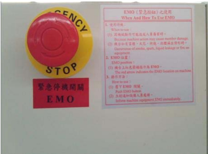
Equipment machine emergency Stop with Chinese and English sign
